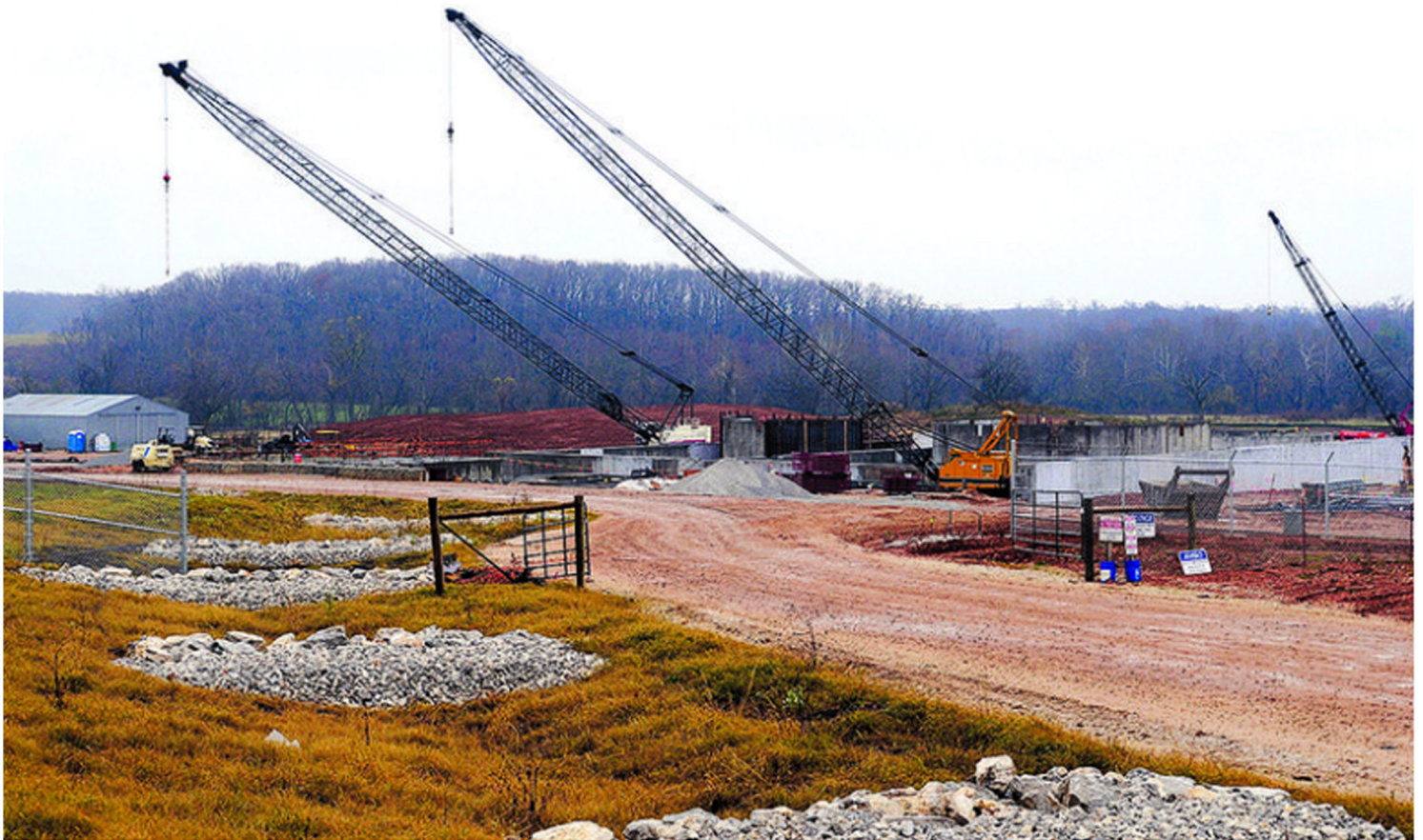
Northwest Arkansas Democrat-Gazette/FILE PHOTO The regional wastewater treatment plant project under construction Friday, Nov. 21, 2009 in Highfill.
