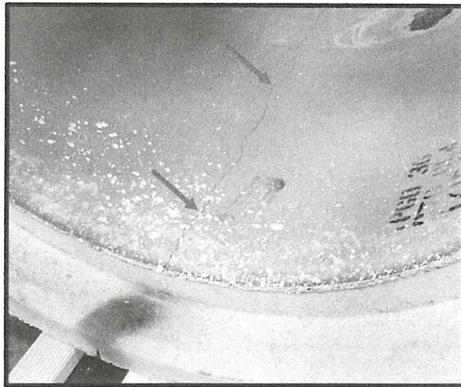
Figure 2 – Inside Crack Example
